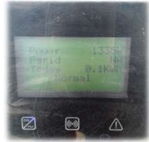
3 kVA Solax make inverter running smoothly via the optimizer.
