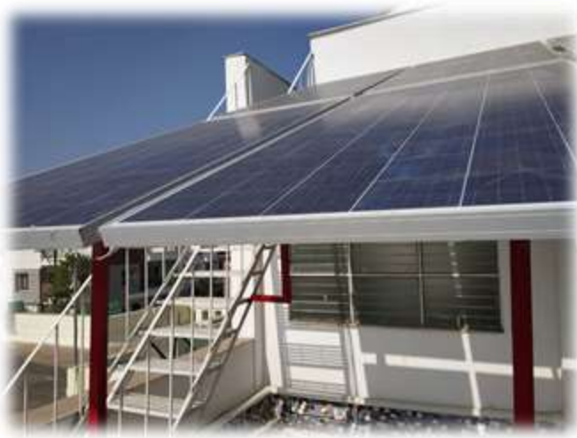
3 kW solar grid connect site photograph at Bhopal.
